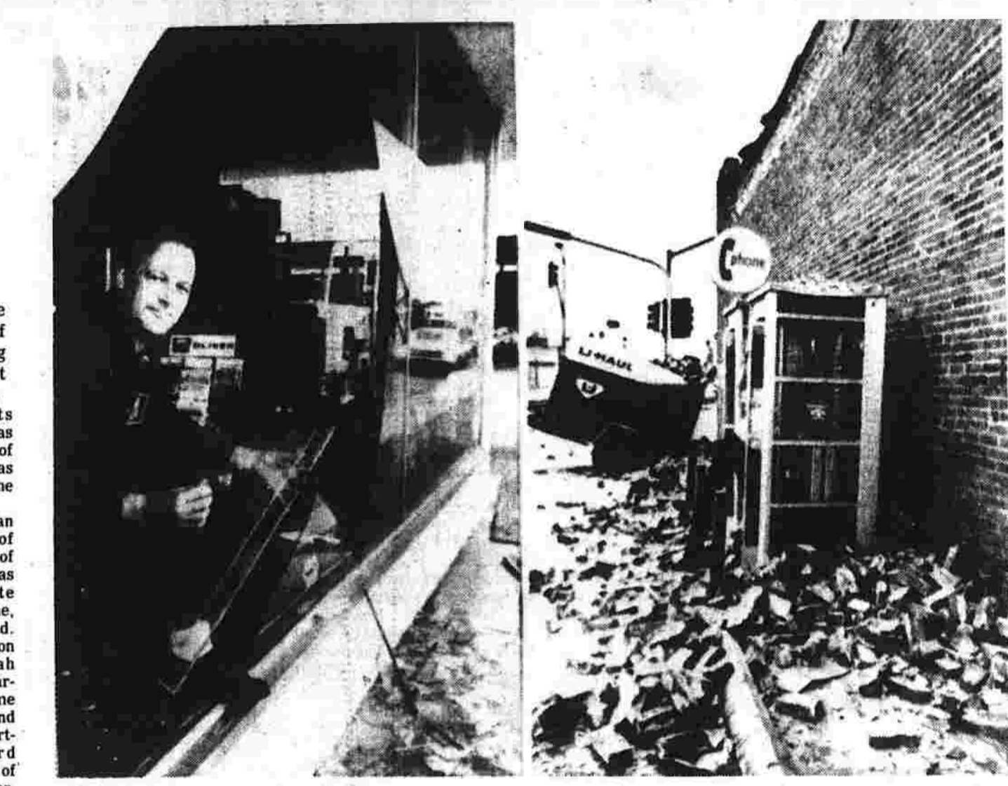
Otto Schless looks through a shattered window at a farm implement store in Oxnard, Calif., Wednesday, where an earthquake centered a jolt felt throughout much of southern California. At right, bricks fell from top of a building onto a telephone booth and a rental trailer. Damage in Oxnard was estimated unofficially at about $1 million. (AP photo)
